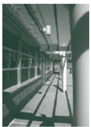
Trellis work protects double glazed window, and adds a distinctive look to Anza.
