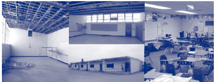
Left and Center (Top): Phase I of the modernizations includes rooms 1-5, and 24, 25 A & B. Center (Bottom): The new permanent modular classrooms are well-liked by teachers. Right: Interior view of one of the new modular units.
